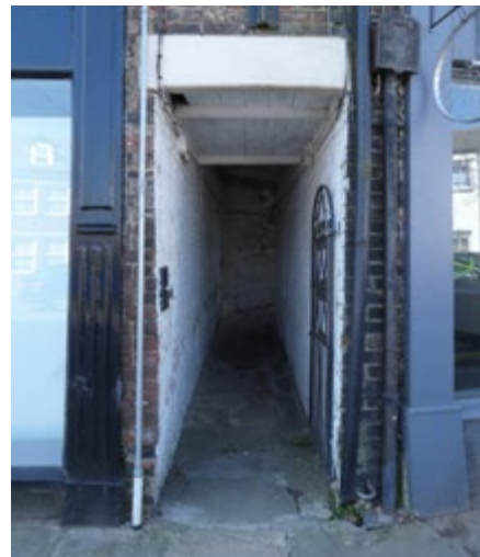
2.20 Typical opening to alley with timber lined soffit and painted brick walls (Insall)
