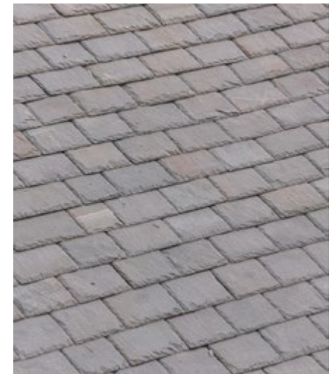
5.3 Natural slates, Wentworth Woodhouse (Insalls).
