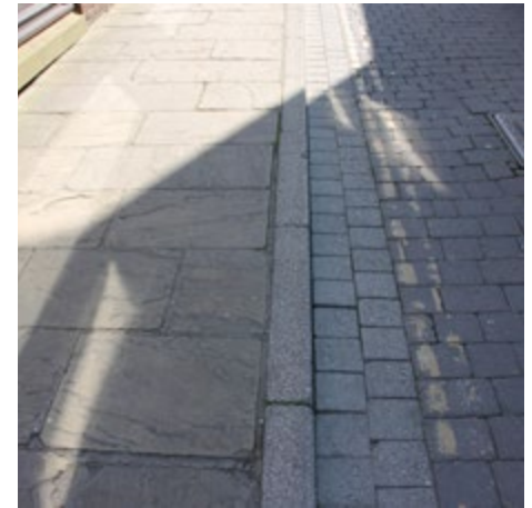
6.8 Yorkstone paving is common to footways and should be retained where possible, on Wren Lane
